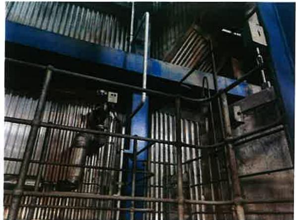
No.2 Soot Floor 3 R
